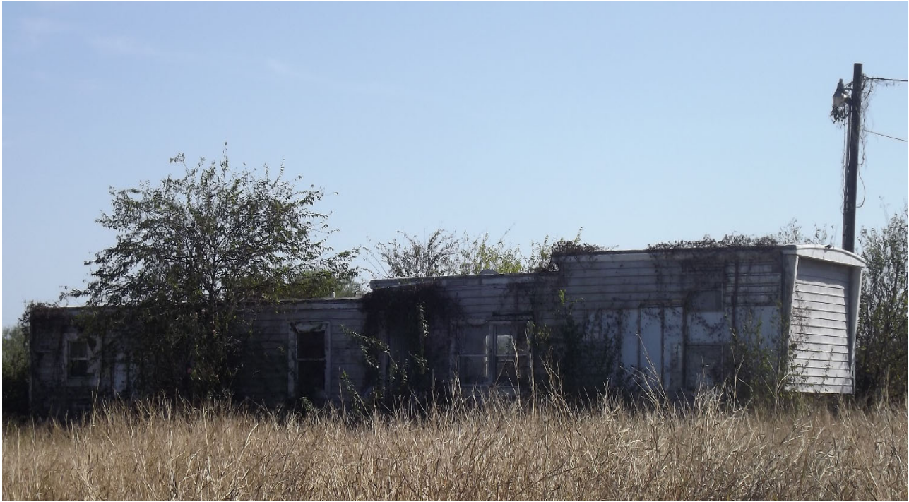
Example of a Single Manufactured Home with graduating step roof and addition
